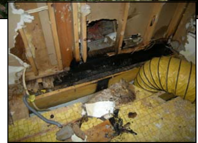
Photos above: Pettyjohn's Cleaning & Restoration/ Water Out Raleigh dry home after fire
