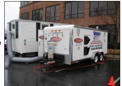
Mr. Rapid hooks up Water Out® Trailer and dries flood house for Encompass presentation in Ohio
