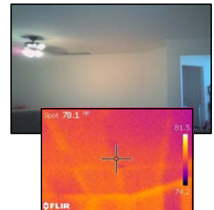
After drying, infrared image and photo show ceiling and wall dry
