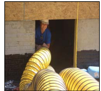
Kelly Cressy of Water Out Coastal helps set up on the Extreme Makeover: Home Edition in Rockville, Maryland
