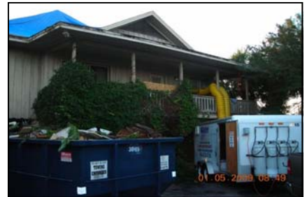
Water Out Northeast Florida sets up their Water Out trailer to dry out after fire
