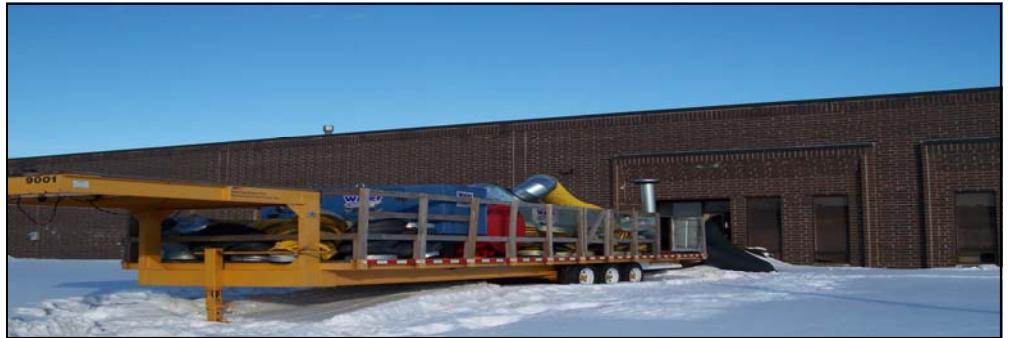
Photo below: Water Out in Libertyville/ Metropolitan Fire Restoration Services using YD9000 to dry 17,000sf commercial building
