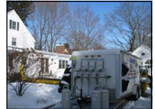
Photos above and below: Water Out in Stormville NY/ Zott Construction dries home in Bronxville, NY
