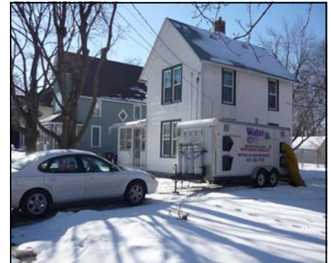
Rainbow International of Quad Cities uses their Water Out trailer to defrost, heat and dry residential home in Illinois
